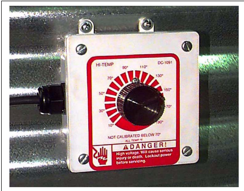
Figure 3E Plenum Thermostat Mounting on Bin Wall
